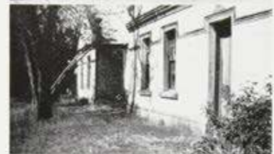
C.1870. CHILDHOOD: A LONG BEDROOM BLOCK BUTTS INTO THE SIDE OF A SECONDARY GABLED WING; NEAR BENDIGO; A FORMER HOTEL ROTS IN DISUSE; THE STONE GABLE END IS SUPPORTED BY THREE GROANING POLES.
