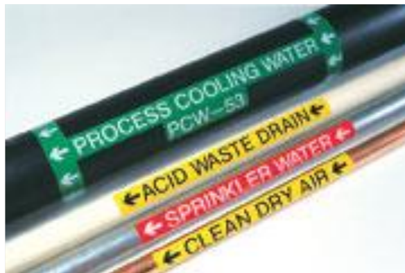
Figure 4 – example of identifying pipework
