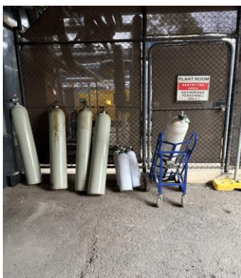
Figure 1: Unsafe gas cylinder storage
