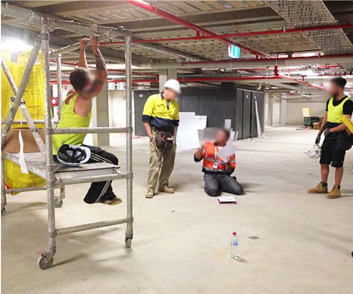
Image 20: the three workers and David – note the ceiling staples, and hanging frame for cabling – the insulation needs to be applied above the frame. Insulation boards in the background
