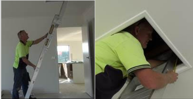
Image 11 and 12: difficulty accessing ceiling manhole using a straight ladder
