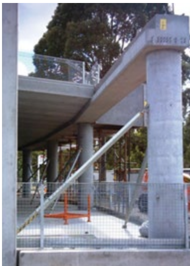
Description: Precast reinforced concrete columns, beams and slab panels. Source: CRC for Construction Innovation
