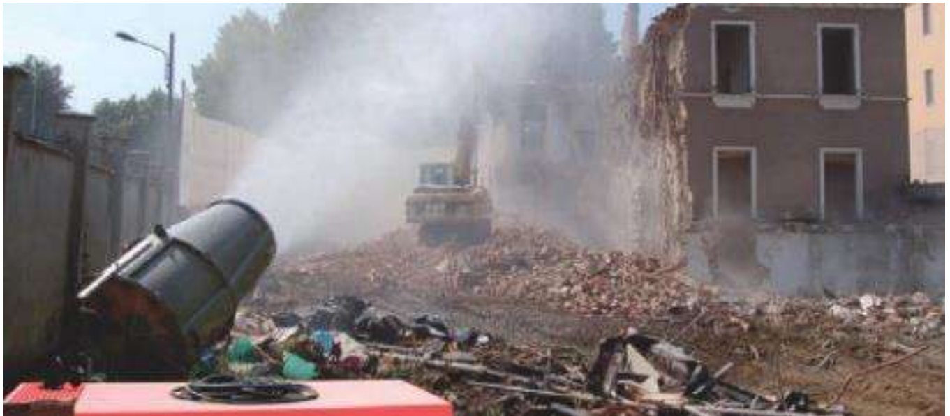
Figure 5.5. Dust suppression using water spray during demolition works (photo courtesy of Kane Constructions).
