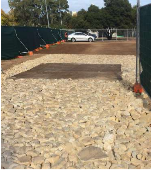
Figure 2. Rumble grid (photo courtesy of McConnell Dowell).
