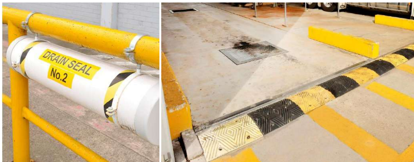
Figure 7.5. Drain seal (left) and rollover bund (right).
