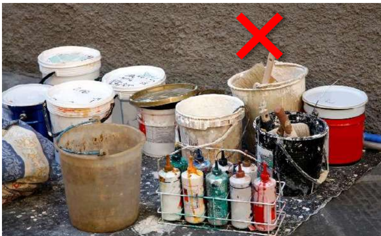
Figure 7.1. Incorrect chemical storage onsite.
